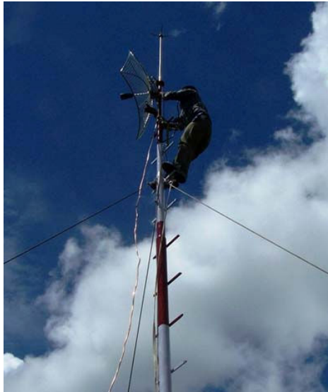
Relay tower at Dip pointing high to Mohare Relay station
