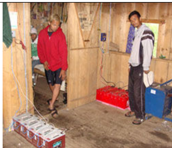
Backup batteries at Mohare Relay
