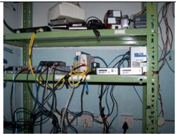
Routers at the server room in Pokhara
