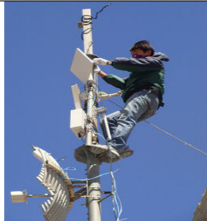
Radios and Antenna at Dhakajung Relay
