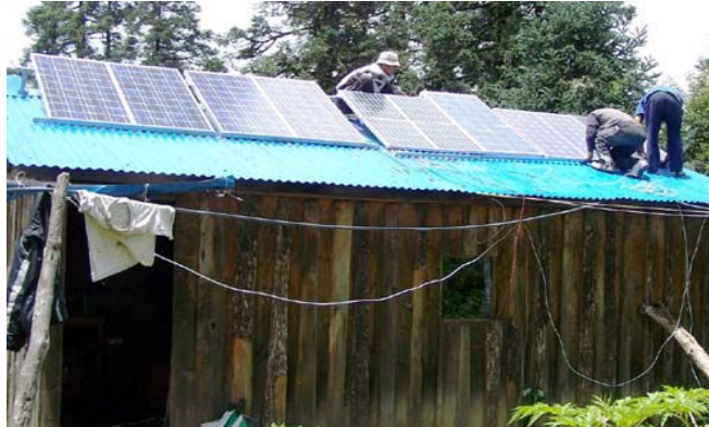
Solar panels at Mohare Relay Station
