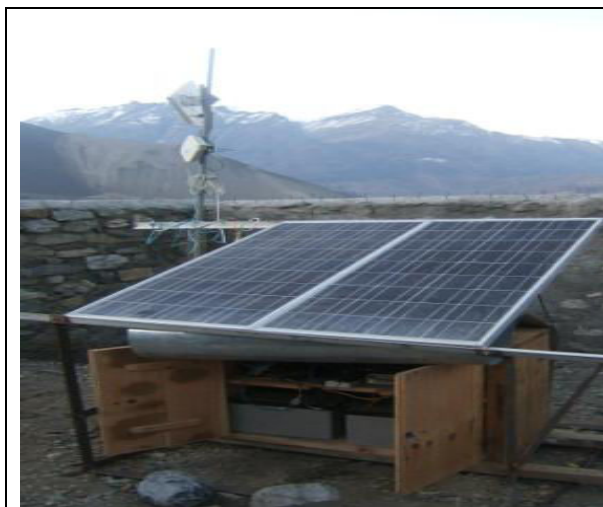
Solar Panels at Kagbeni Relay
