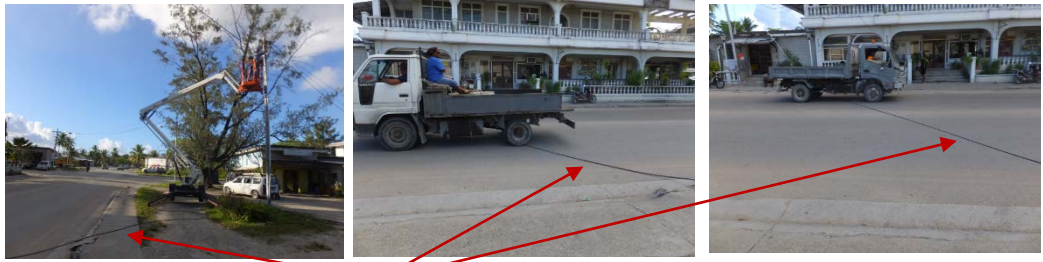
Optical fiber cable on the road due to not stop the traffic during holing cable.
