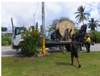
Due to limited time of truck rental Roll down the cable on the road carefully seeing the small sharp stone
