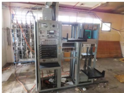
Fore Past equipment room
