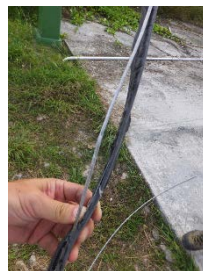
2 day ago, in very hot day, we found cable was damaged due to high temperature and traffic.
