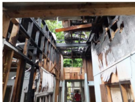
Some years ago, Kids fired the building
