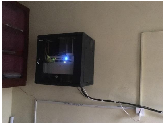
Figure 45: APT Dullu Project Data Center
