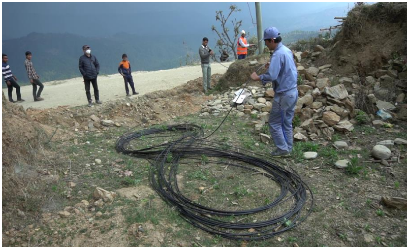
Figure 43: Creating Figure-8 Cable prior to layout (Mr. Ishikawa and Mr. Goto from OCC)
