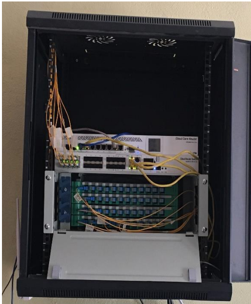
Figure 17: APT Dullu Project Data Center (Optical Router/Switch/Patch Panel)
