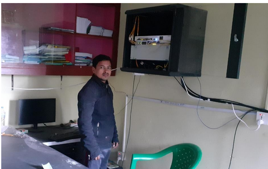
Figure 47: Dullu Municipality Technologist, Mr. Nirajan Hamal. Currently pro-bono contribution of managing network in post- project handover phase.
