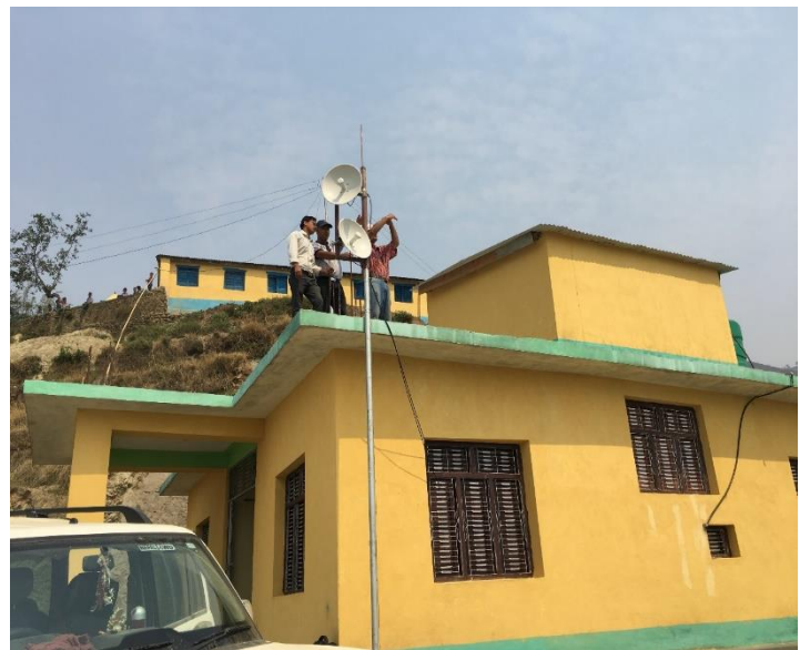
Figure 20: Dullu Municipality, Ward 1 Wireless Point to Point Relay Install
