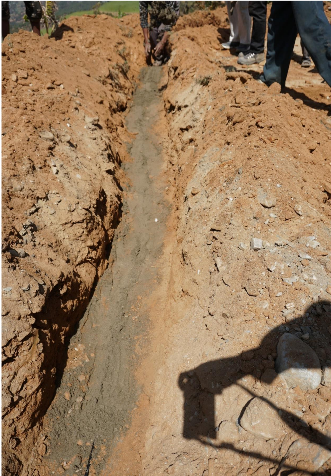
Figure 32: Manual OFC Layout (clearing of rocks and pebbles, laying of soft sand around the OFC, and refilling with original/native soil
