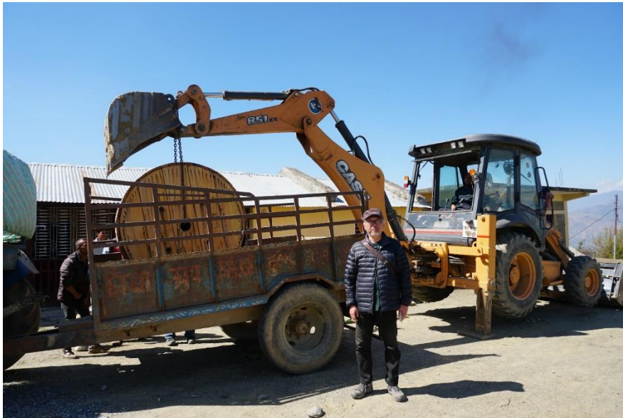
Figure 38: OCC Optical Fiber Cable Drum being transported from storage to installation sites
