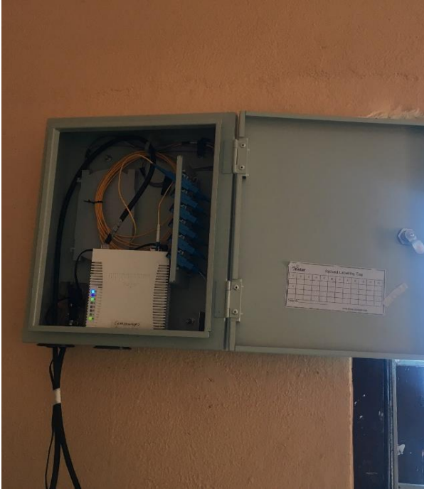
Figure 19: CPE Fiber Terminal Box
