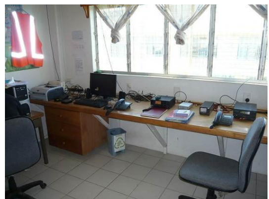
Figure 4.1 Communication room in NEMO
